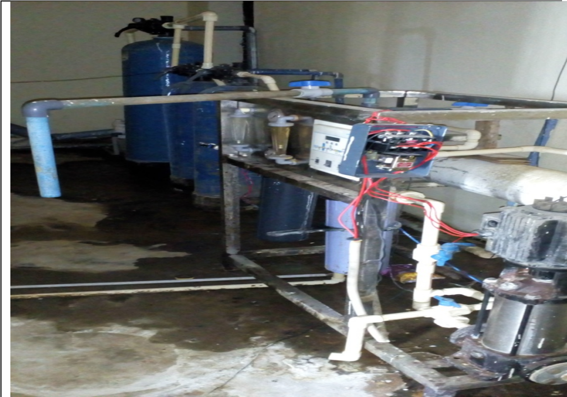
RO Mineral Water plant
