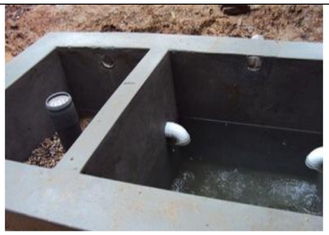
Water collecting system
