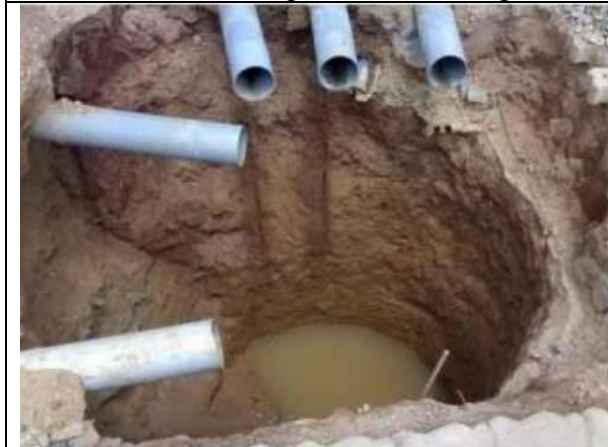
Water collecting system
