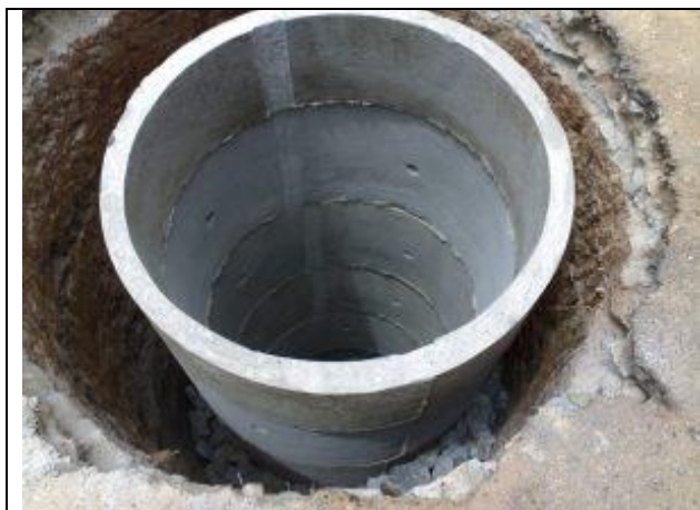
Rain water harvesting water collecting tank
