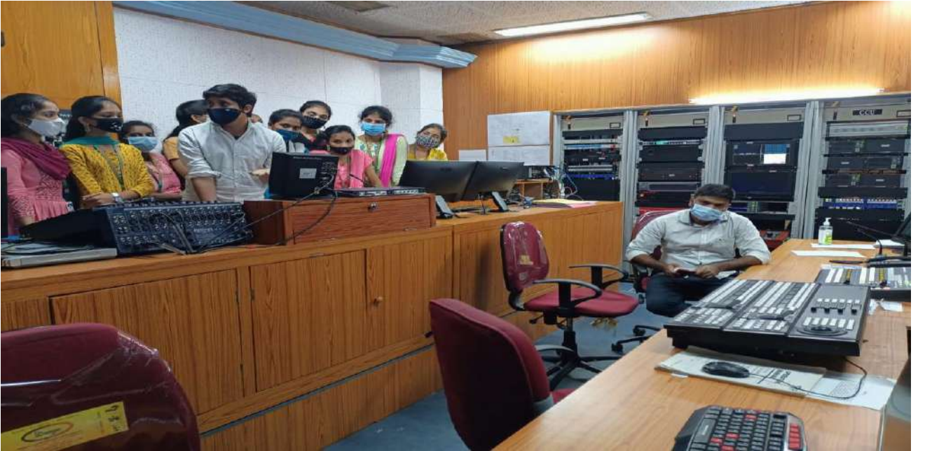
Photos: Doordarshan Kendra Vijawada Video and Audio Processing Units ,High Power Earth station Transmitter unit
